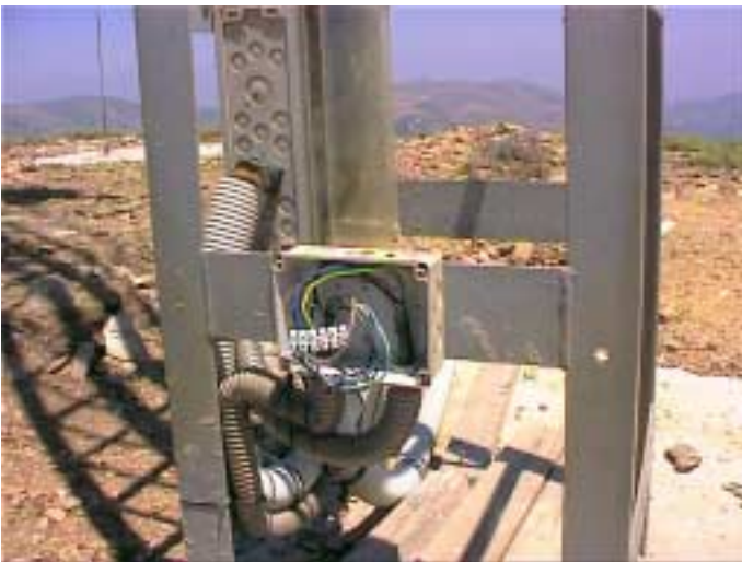
Figure 13 : Terminal box at the WTG
