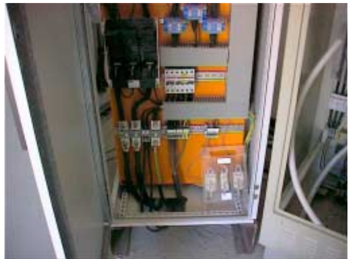
Figure 17: Cable – entrance to the DC/AC- converter (PV system module 1)
