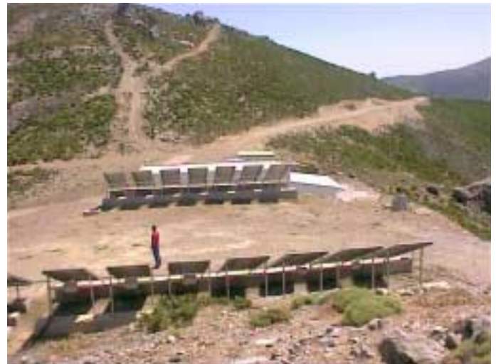
Figure 7: PV – system modules 1 and 3 in front of the electrical station
