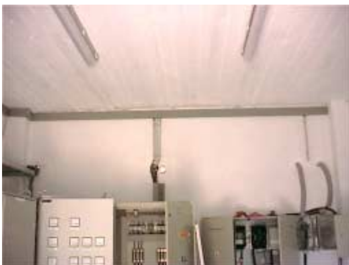
Figure 16: Entrance of the cables and wires in the electrical station (left: PV-systems; middle: appartement house/cold-storage house; right: WTGs and biogas-system)
