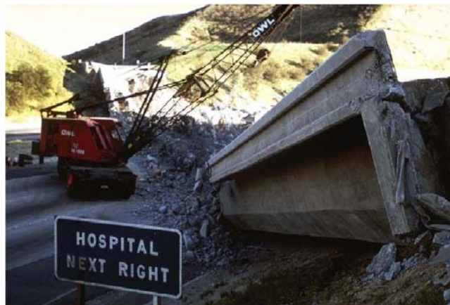
Figure 1: Collapsed bridge impeding traffic to hospital resulting from 1971 San Fernando Earthquake [3].
